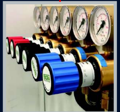
Pannello controllo gas Gas distribution manifold
